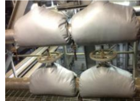
Steam Line Insulation Jackets
